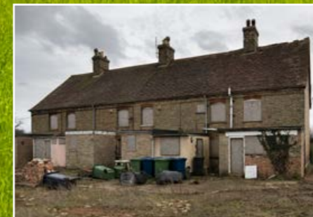
Former farm workers cottages in Gamlingay, Bedfordshire have been fully refurbished and extended to provide modern, contemporary homes.
